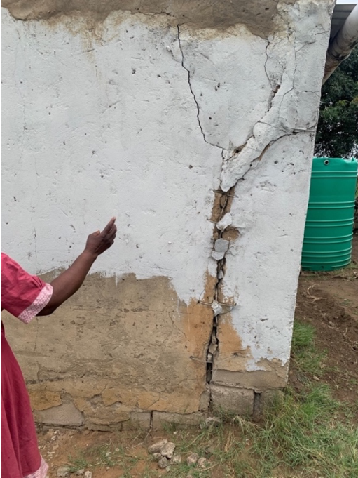
Image 6. Damage attributed to blasting ( Photo credit: Garret Barnwell, 2022 )
