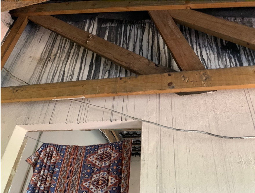
Image 8. Roofs bleed black. (Photo credit: Garret Barnwell, 2022).
