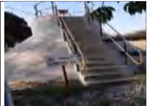
Anaerobic digesters for sludge treatment is not operational and sludge is spillage to the surrounding environment
