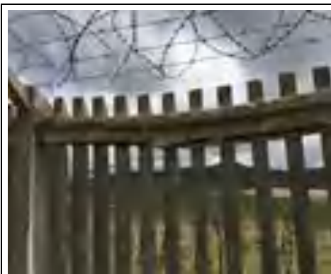
The palisade fence in a state of disrepair
