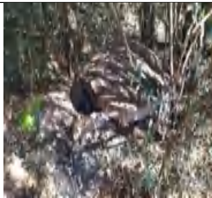
Leakage in sewer network
