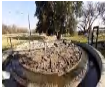
Settling of sewage is severely compromised by non-operational equipment and lack of process control
