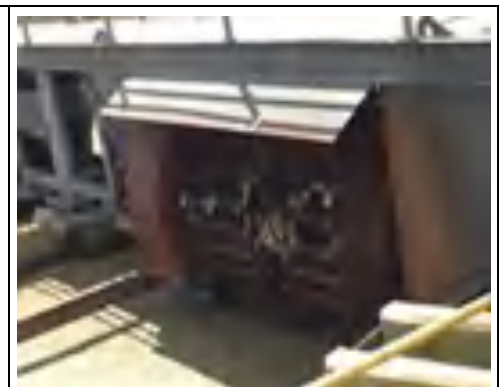
1 of 2 aerators are dysfunctional in the Pasveer ditch
