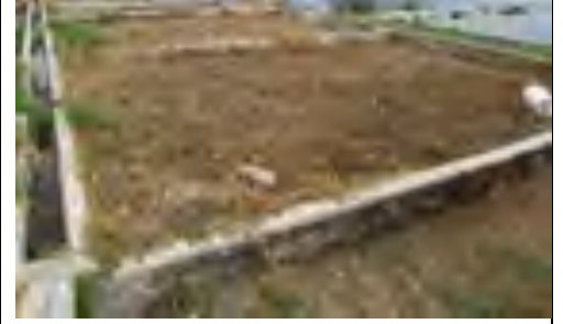
Ponds not well maintained, plant growth on structures, terrain reasonably well maintained on the terrain
