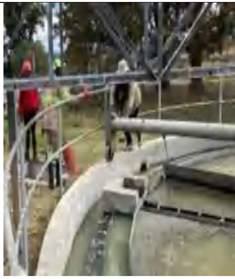
PSTs not operational - operators have to manually push scum trap arm; no motors to drive the arm
