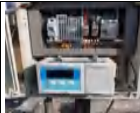
Flow meter is in place and functional, but data is not interpreted and reported against design capacity
