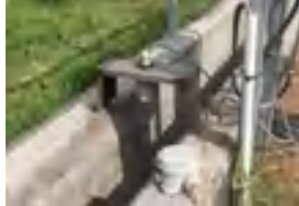
Grit removal is functional, but overloaded due to excessive grit entering the site
