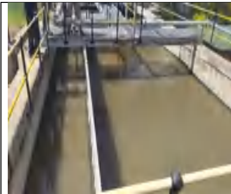
Sludge withdrawal dysfunctional
